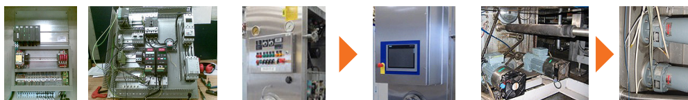
PLC and electrical components mounted on backplate
